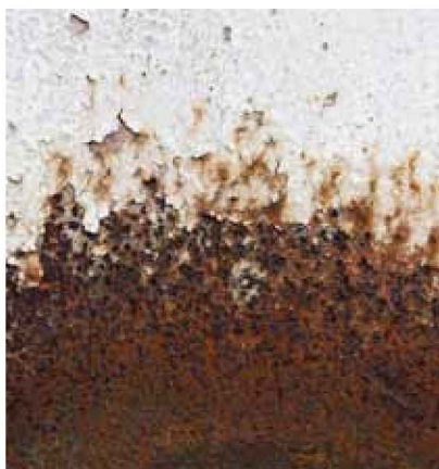
Rust forming on painted steel
